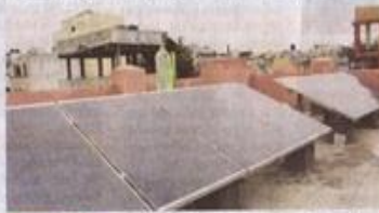
Not more shikha: Solar panels set up by 4FPL at Government Primary School, new Bholguda, Secunderabad, have helped the school save on power bills
